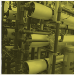
Wastewater and Sewage Treatment
