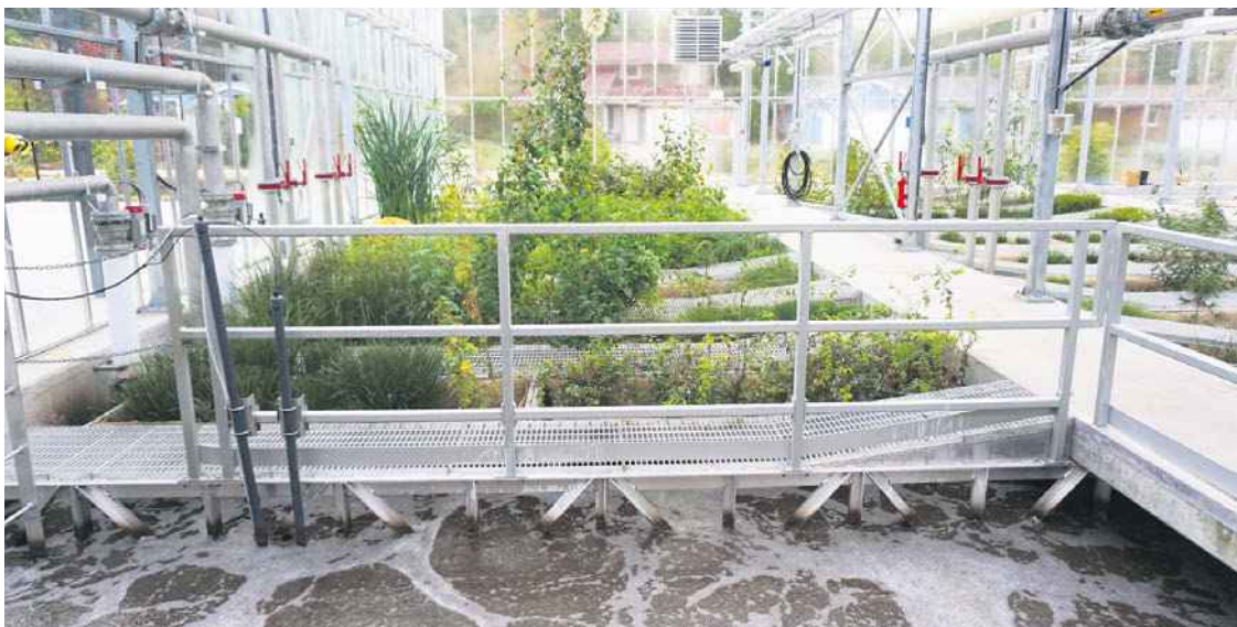
Technology developed by International Wastewater Systems recovers the heat generated by sewage to meet the heating and cooling requirements of residential, commercial and institutional buildings, including Sechelt's sewage treatment plant on B.C.'s Sunshine Coast. SUPPLIED
